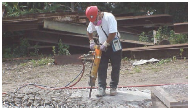
A worker chips concrete with a jackhammer using a water-spray attachment to control dust.
