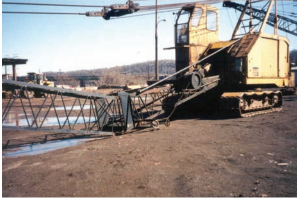
Figure 7. Boom collapse during crane disassembly.
