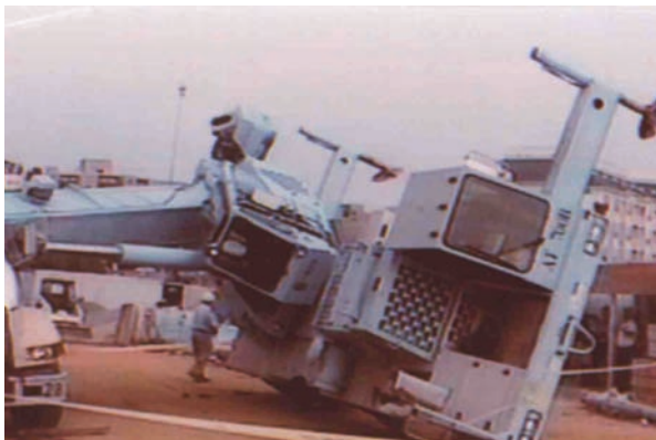
Figure 4. Crane tip-over at construction site. Note that the right outriggers were set, but not extended. (Photo courtesy of OSHA)
