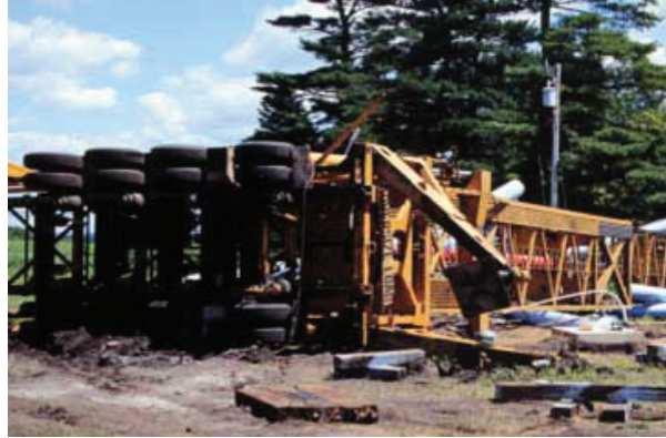
Figure 6. Mobile tower crane tip-over attempting to hoist water tank. (Photo courtesy of Iowa FACE Program)
